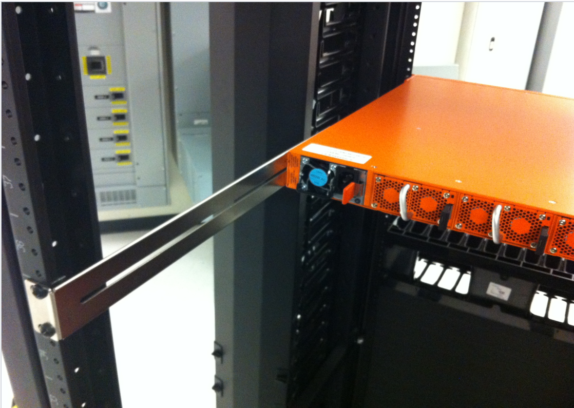
Figure 4: Rear View of the Mounted Node and Rails on the Four-Post Rack
